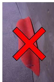
Fig 5 improper fastening to a concave wall
