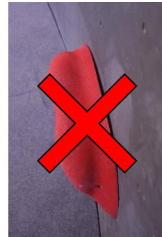
Picture 22 improper attachment at concave wall
